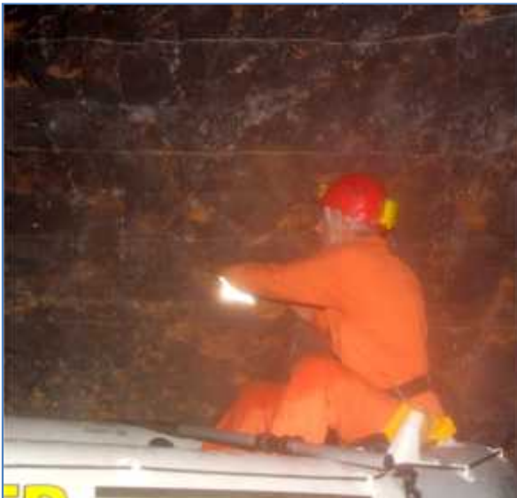
Figure 11. Calcite lines on the cavern walls above the May 2014 water level.
